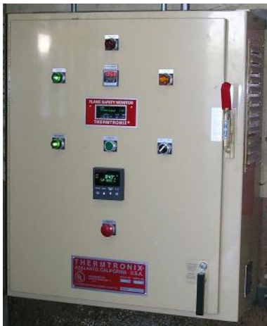
FLAME SAFETY CONTROL GAS FIRED FURNACE
